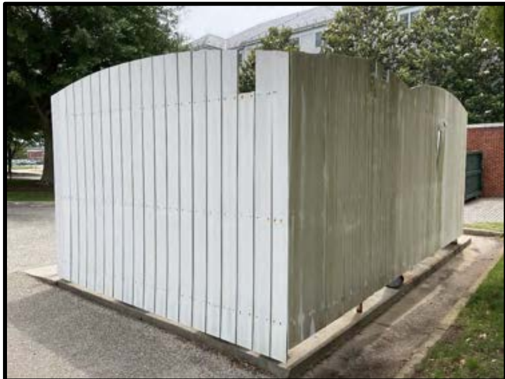
Photo #2: Damaged secondary containment
