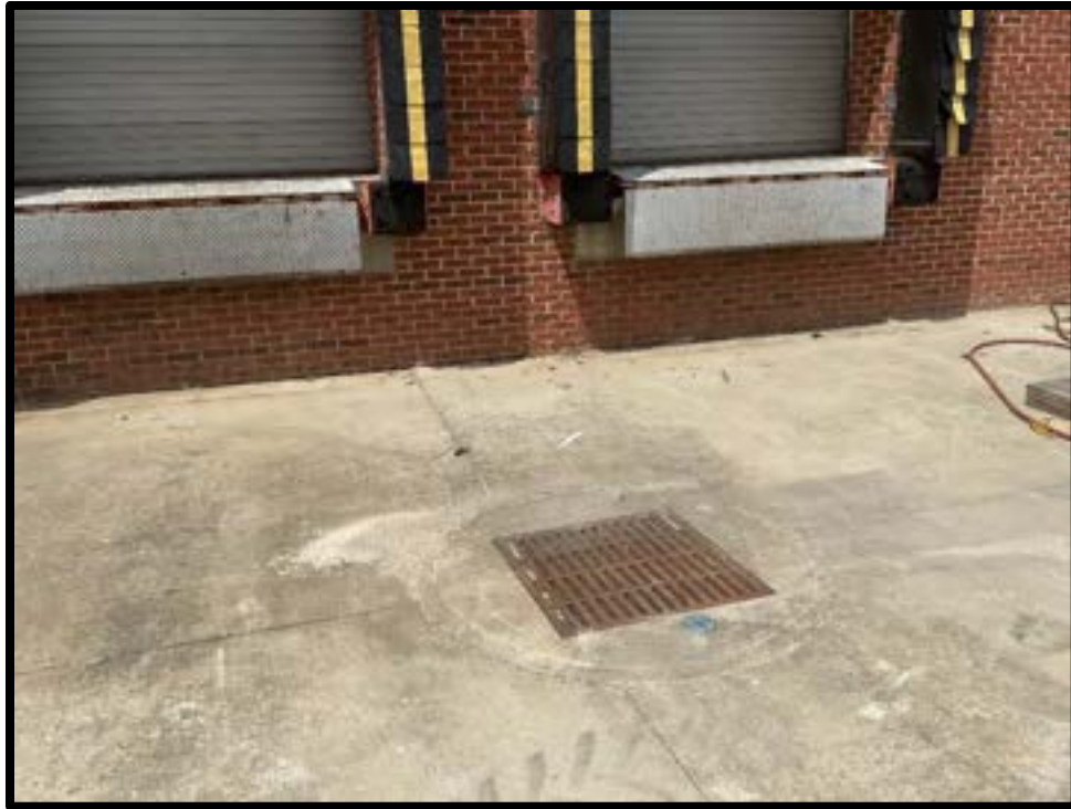
Photo #2: Petroleum smell from first inlet
