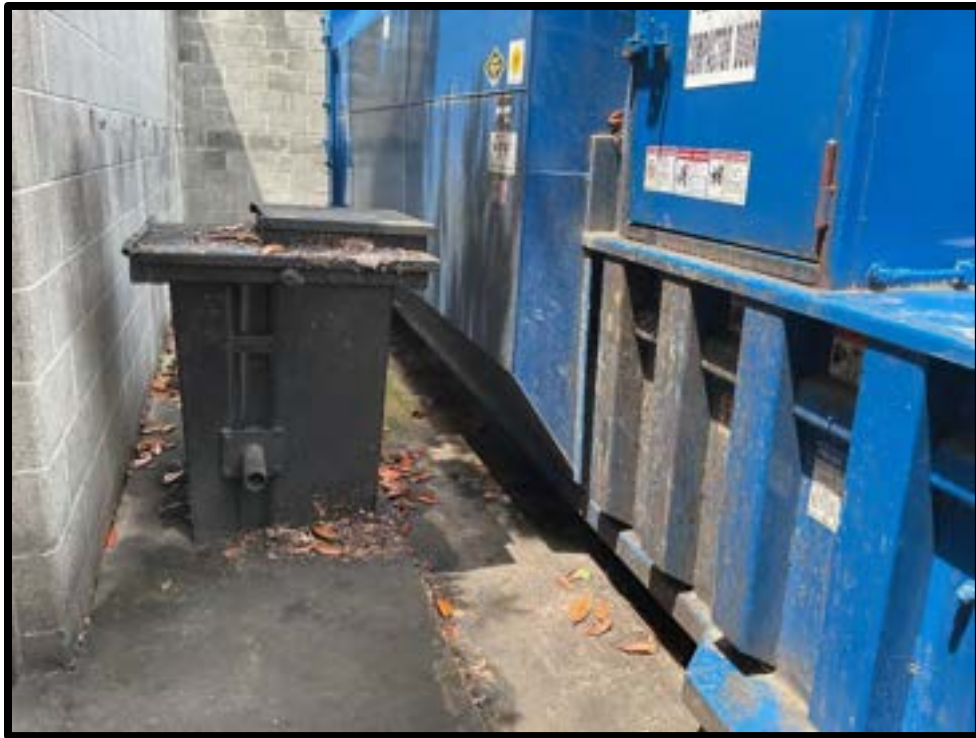
Photo #1: Staining around grease trap and trash compactor
