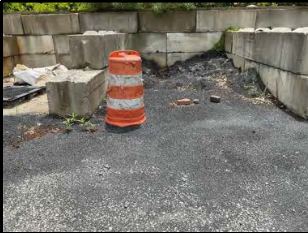
Photo #2: Uncovered stockpile
