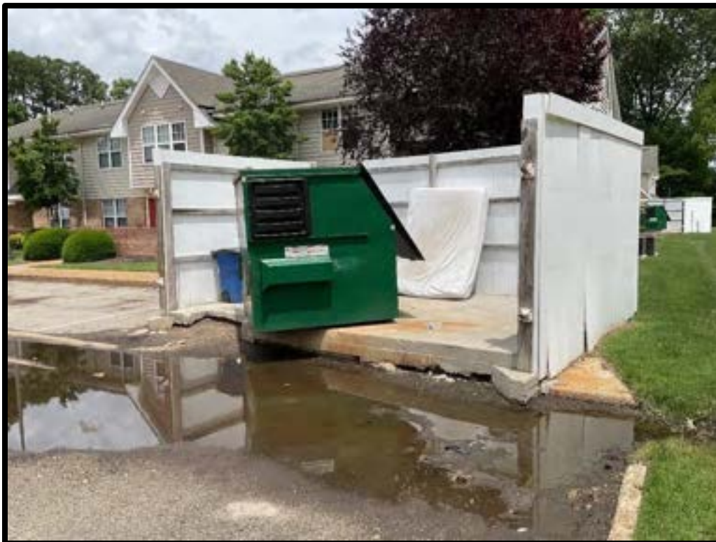
Photo #1: Significant ponding outside of secondary containment
