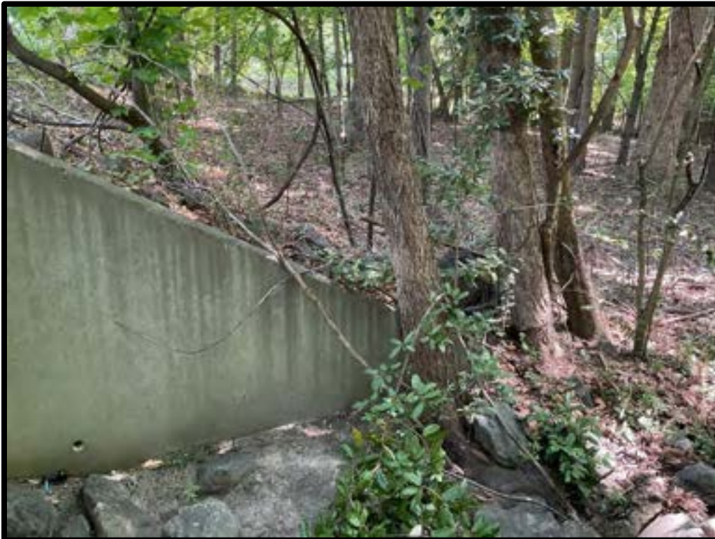
Photo #4: Tree growing into headwall
