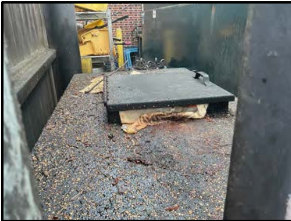
Photo #4: Leaking grease trap
