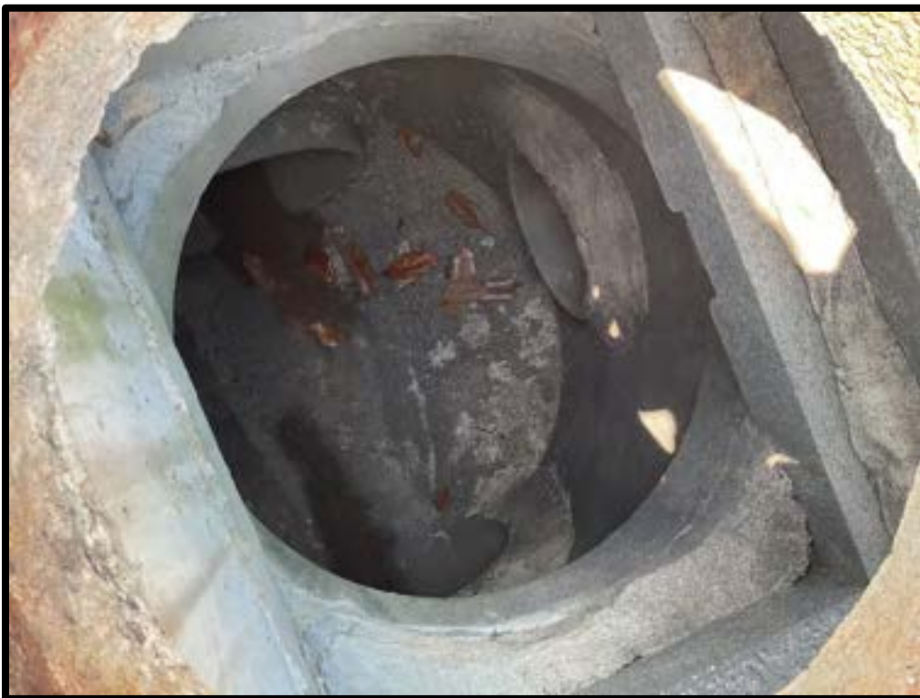
Photo #2: Some sediment and debris accumulation present
