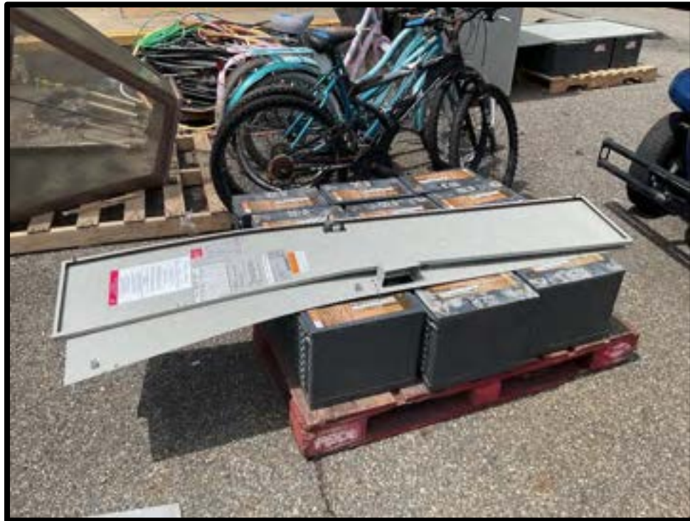
Photo #6: Uncovered batteries
