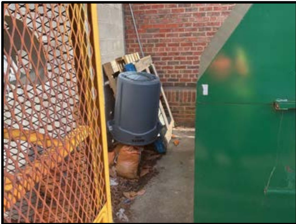
Photo #2: Accumulated Debris
