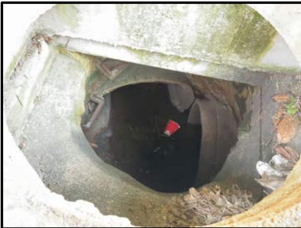
Photo #2: Standing water and debris present
