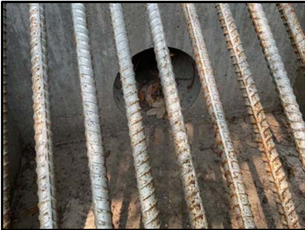
Photo #9: Some debris accumulation present in outlet structure
