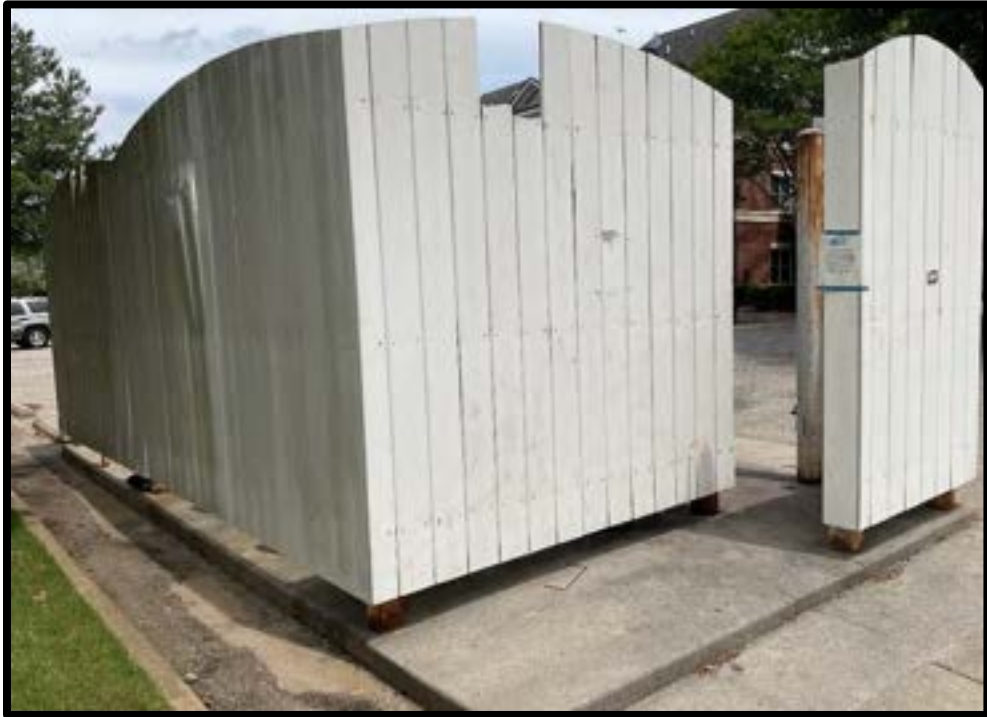
Photo #3: Secondary containment does not reach ground, Educational signage present
