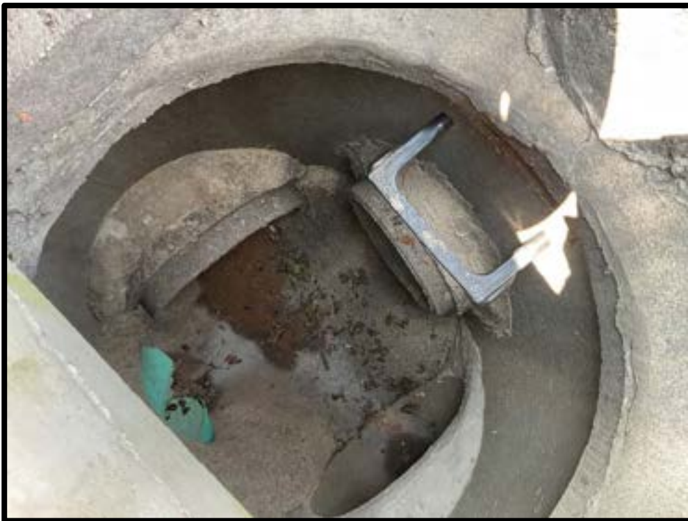
Photo #2: Some debris accumulation present
