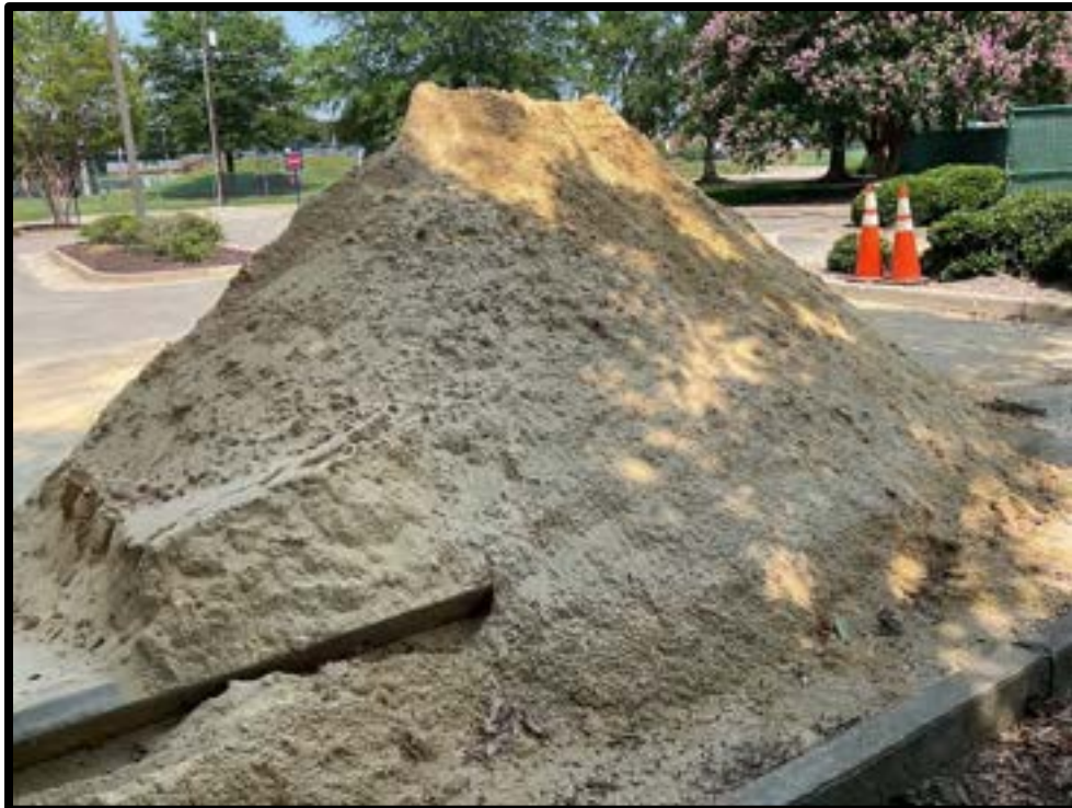
Photo #4: Uncovered stockpile
