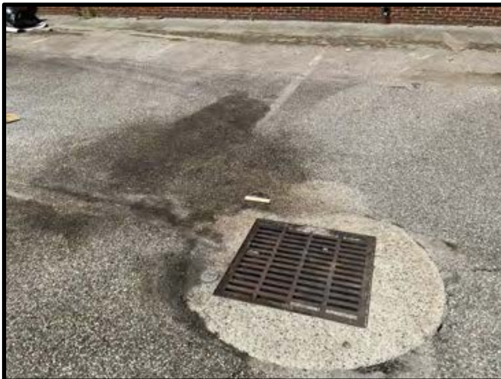
Photo #3: Petroleum stains around second inlet
