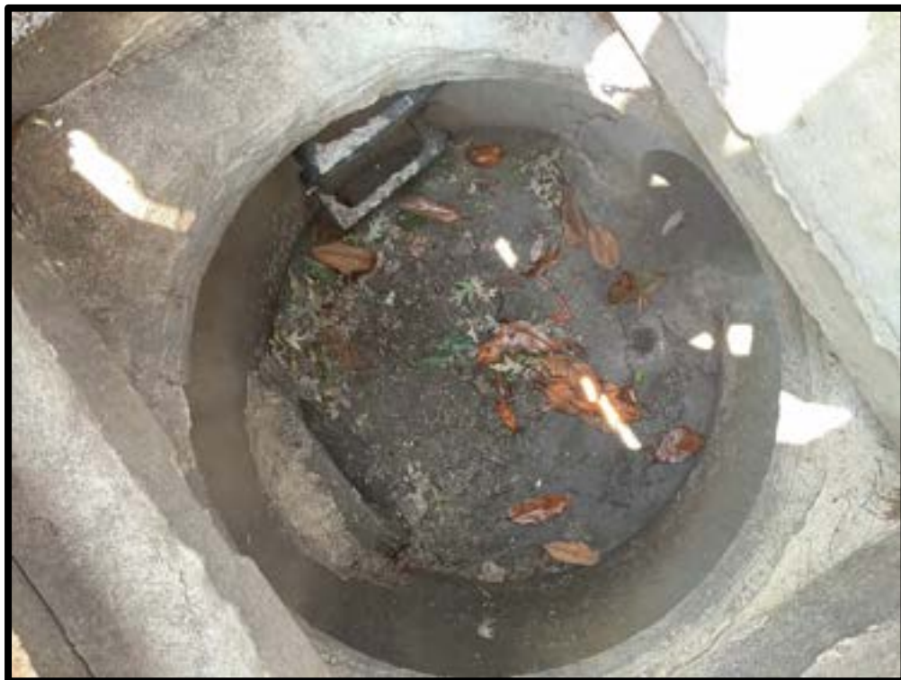
Photo #2: Some sediment and debris accumulation present
