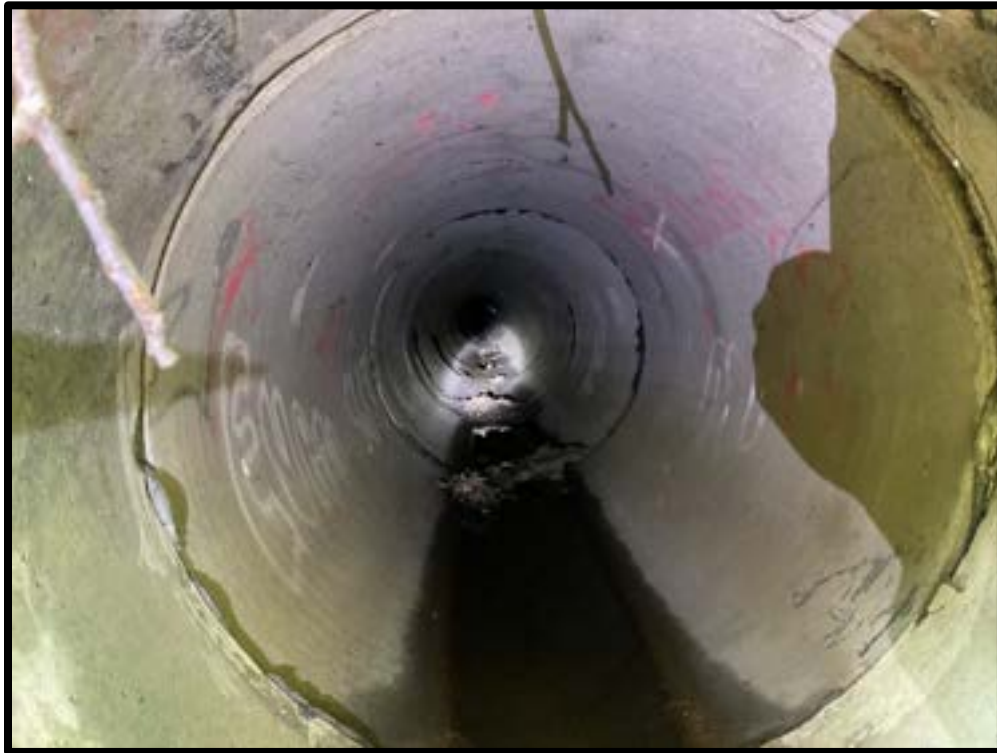
Photo #3: Some debris accumulation in pipe, pipe may be disjointed
