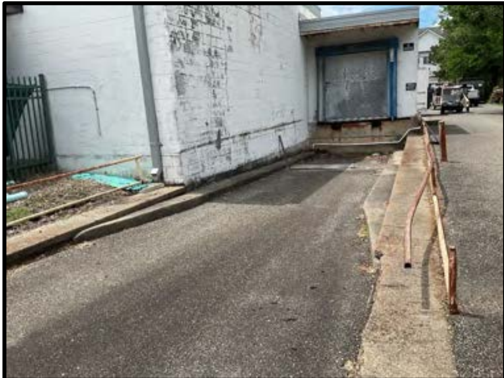
Photo #13: Loading dock and debris accumulation
