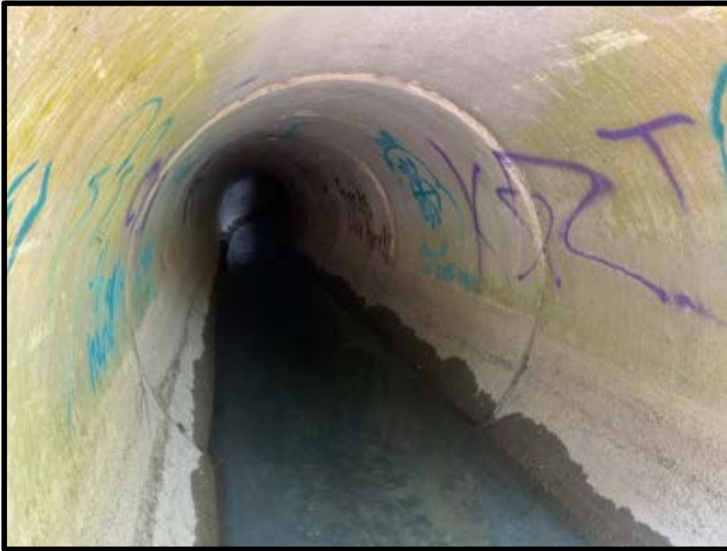
Photo #3: Backwater present in pipe due to receiving channel conditions
