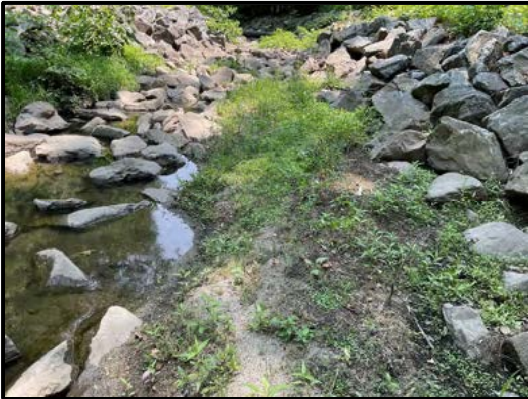
Photo #3: Sediment accumulation in receiving channel
