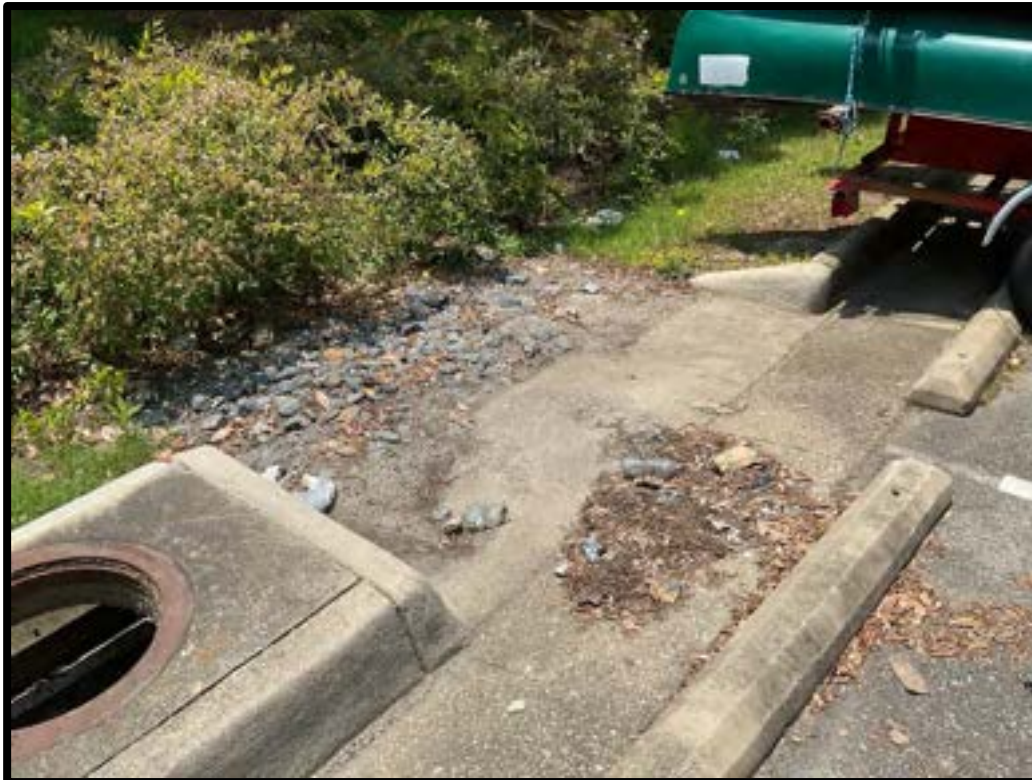
Photo #3: Debris and road grit accumulation present in northern curb cut inlet
