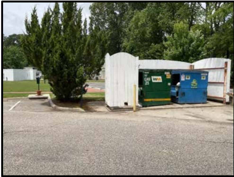
Photo #2: Secondary containment does not reach ground
