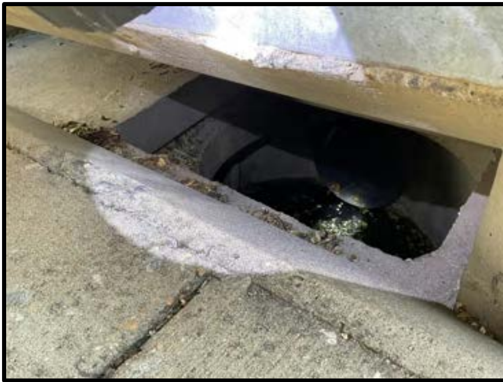
Photo #1: Some debris accumulated in inlet
