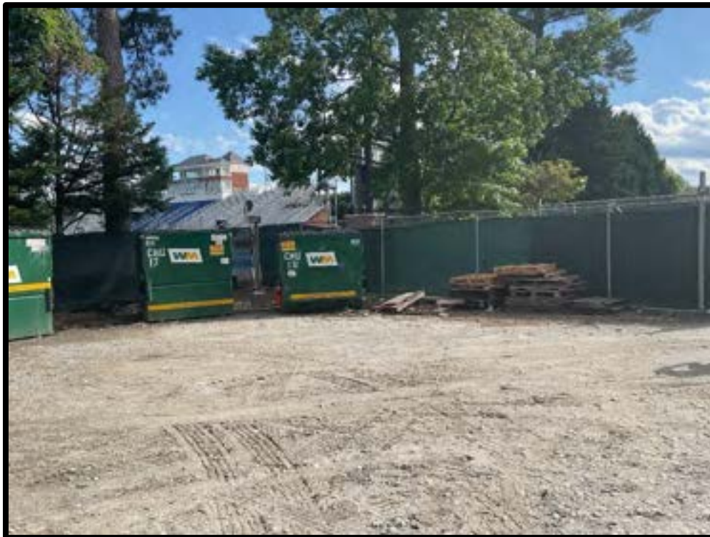
Photo #4: Materials storage and debris accumulation in receptacle area
