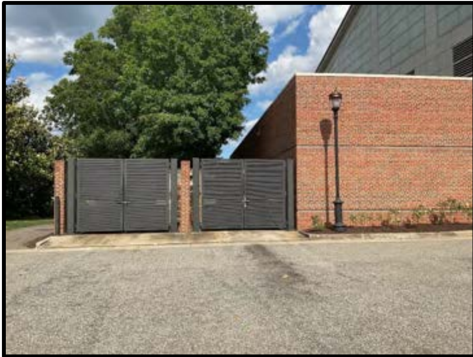
Photo #1: Staining on pavement
