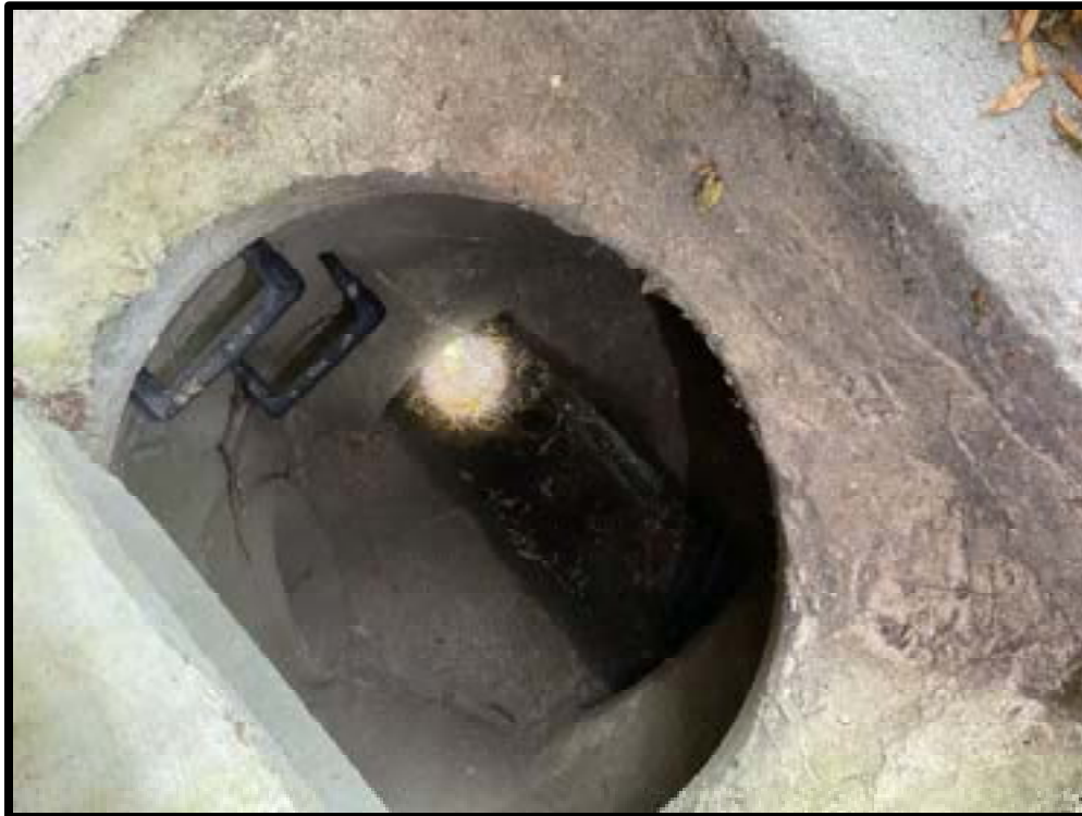
Photo #2: Sediment accumulation present
