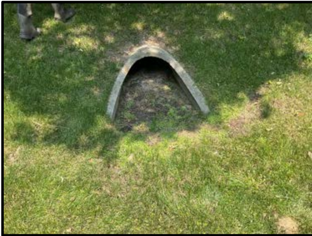
Photo #7: Sediment and vegetation accumulation present in eastern inlet pipe
