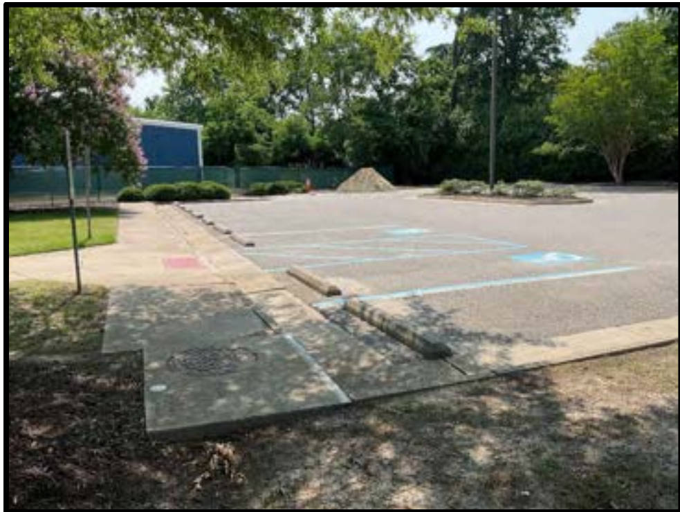
Photo #2: High risk inlet
