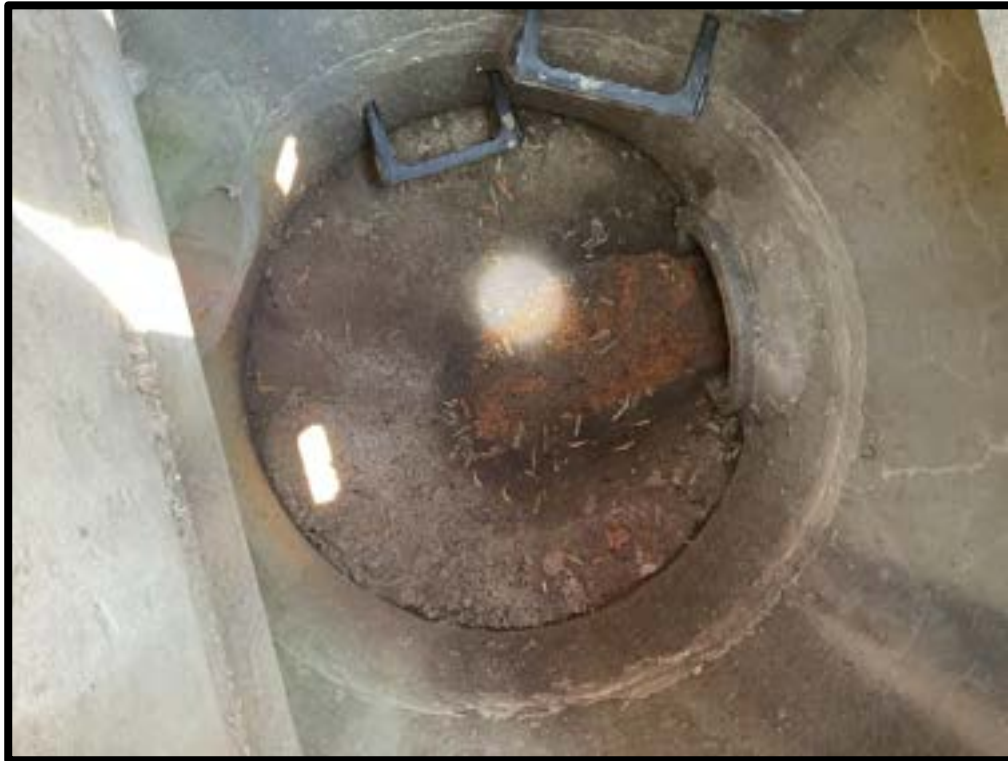
Photo #2: Some sedimentation and debris accumulation present
