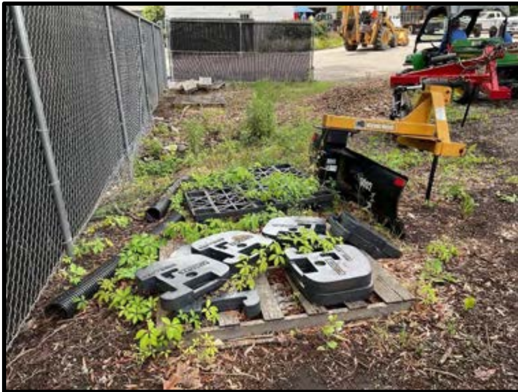
Photo #8: Uncovered materials storage
