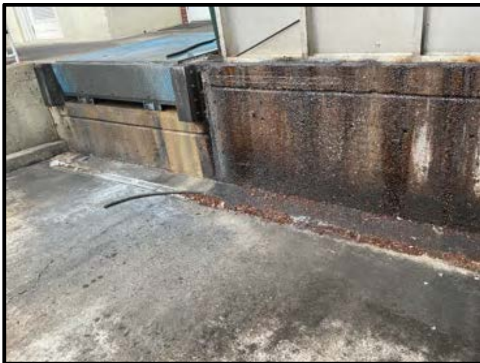
Photo #2: Debris accumulation at trench drain
