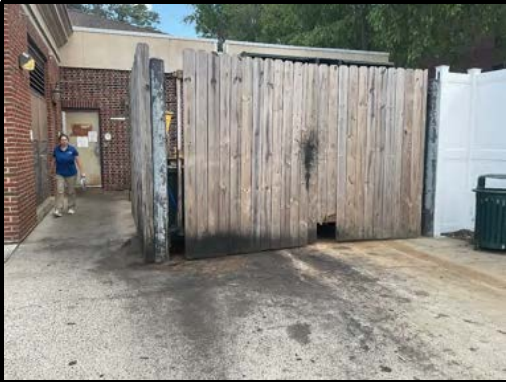
Photo #3: Staining present and damaged secondary containment
