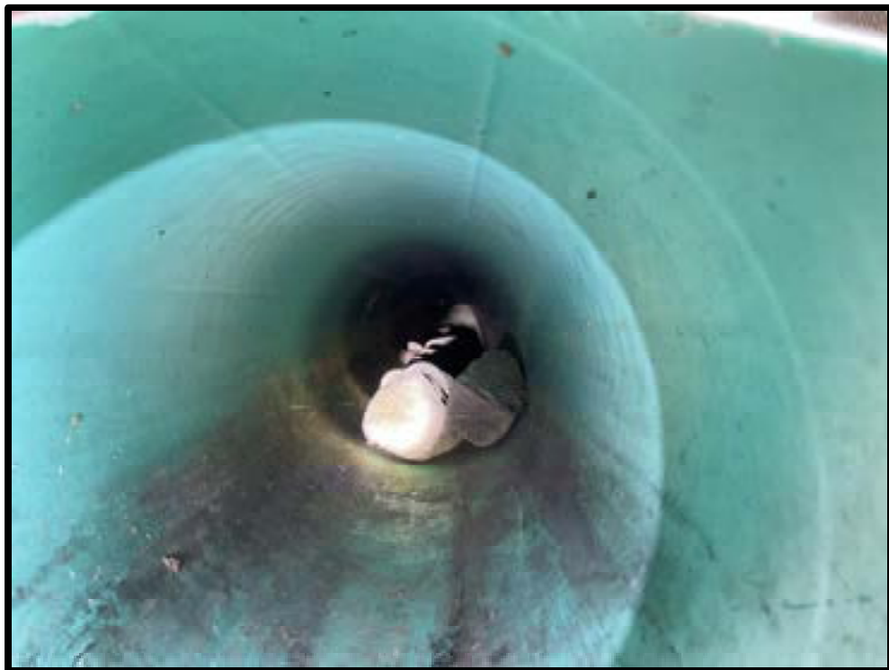
Photo #3: Stones present in western inlet pipe
