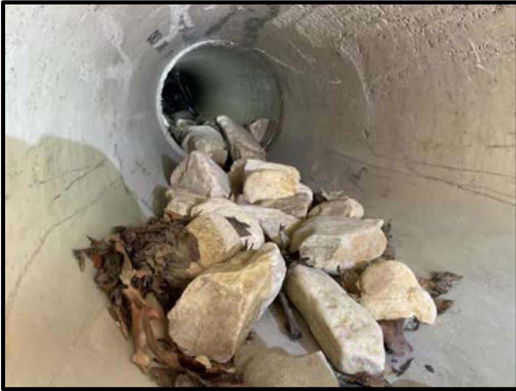
Photo #6: Stones present in northern inlet pipe
