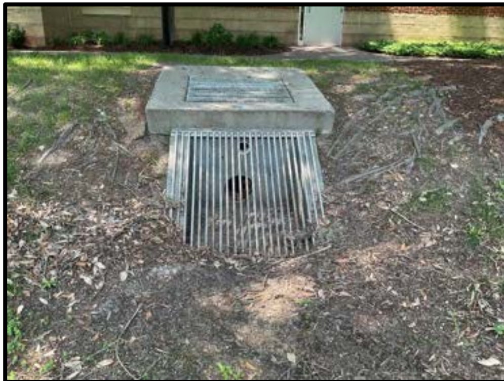
Photo #8: Minor debris accumulation present in outlet trash rack, minor bare areas around outlet structure
