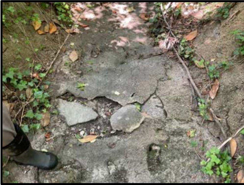
Photo #5: Cracking of receiving channel grout
