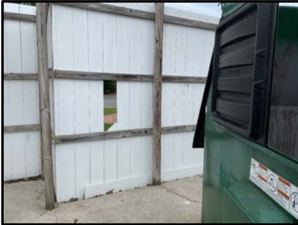
Photo #3: Damaged secondary containment
