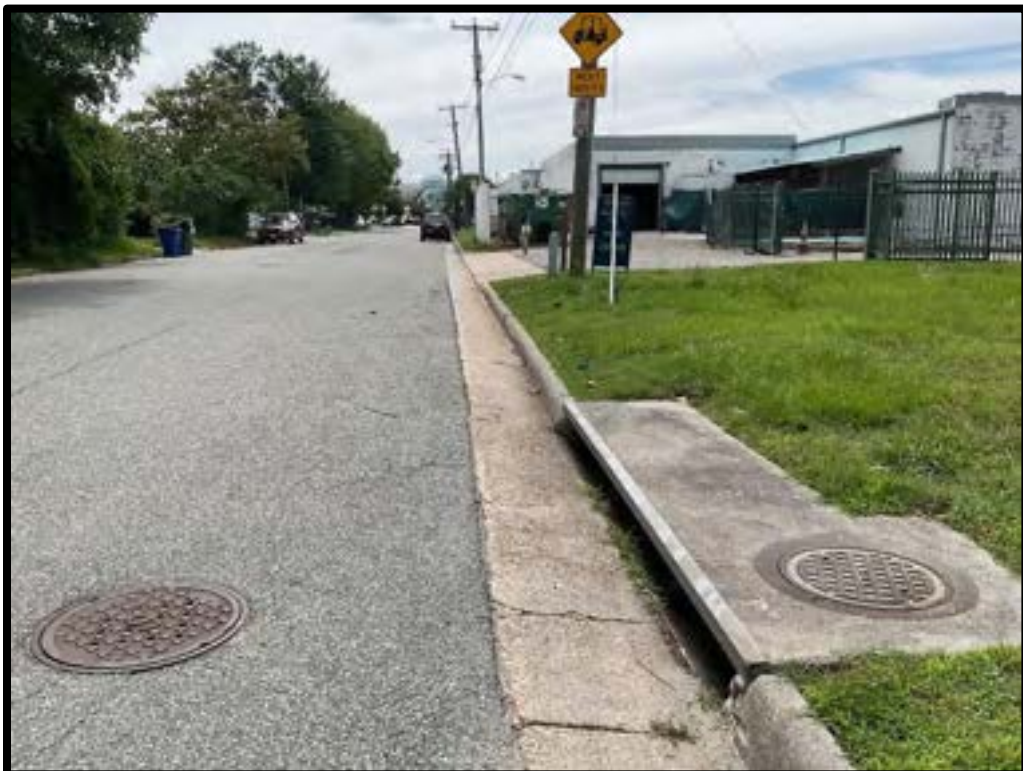
Photo #11: Inlet downstream of leaking dumpster
