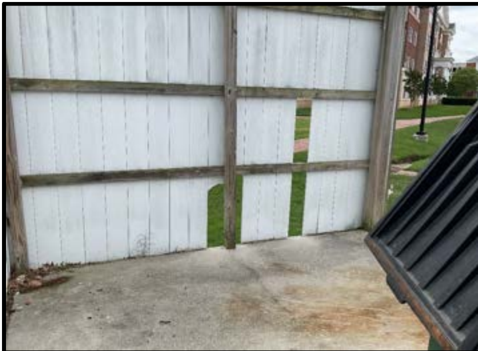
Photo #2: Damaged secondary containment
