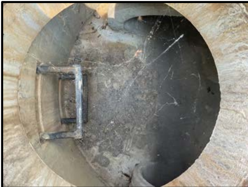
Photo #2: Upstream outfall pipe, sedimentation present
