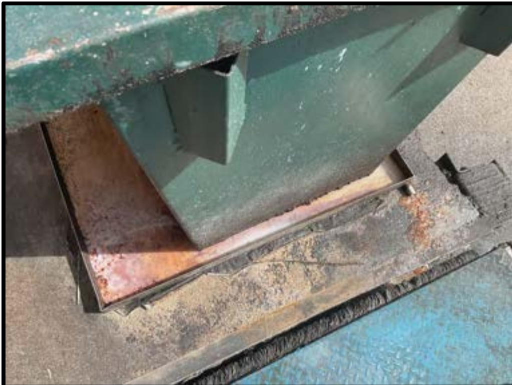
Photo #4: Grease trap secondary containment full of grease and water
