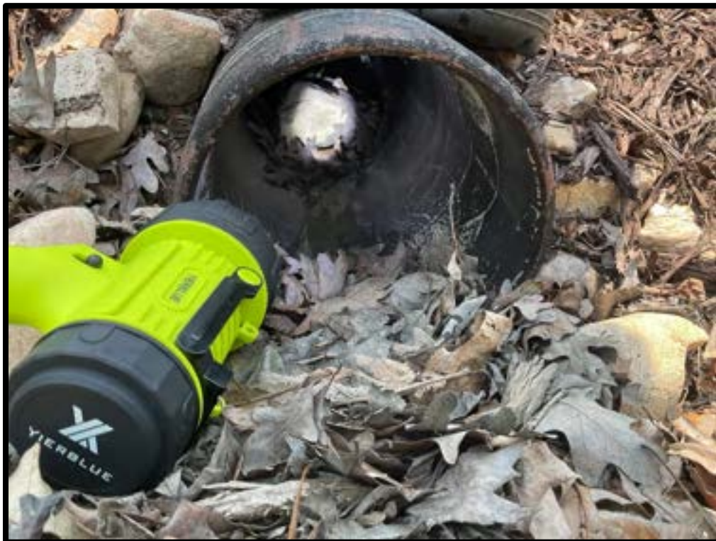
Photo #5: Stones present in southwest inlet pipe
