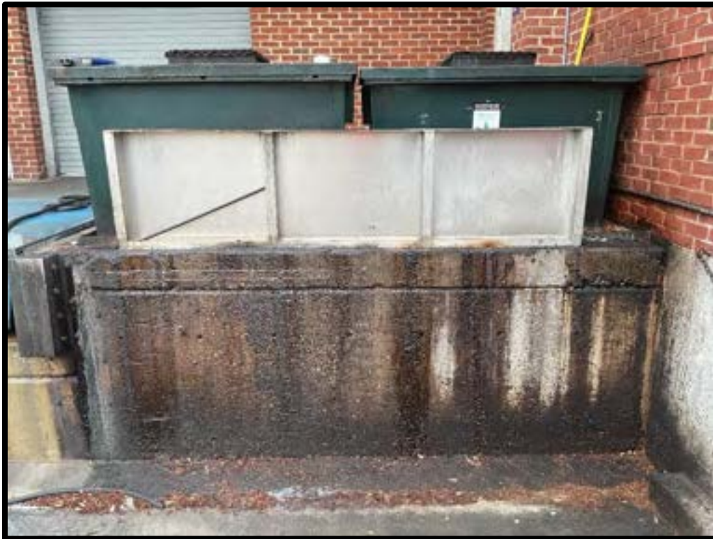
Photo #3: Grease trap leaking and staining
