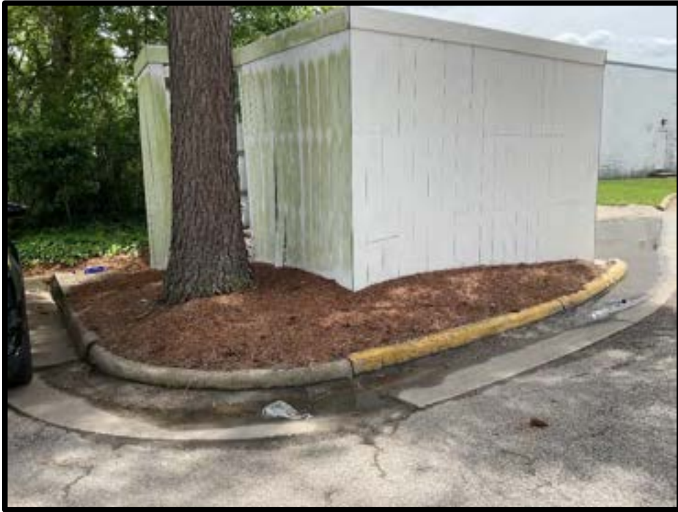
Photo #2: Damaged secondary containment
