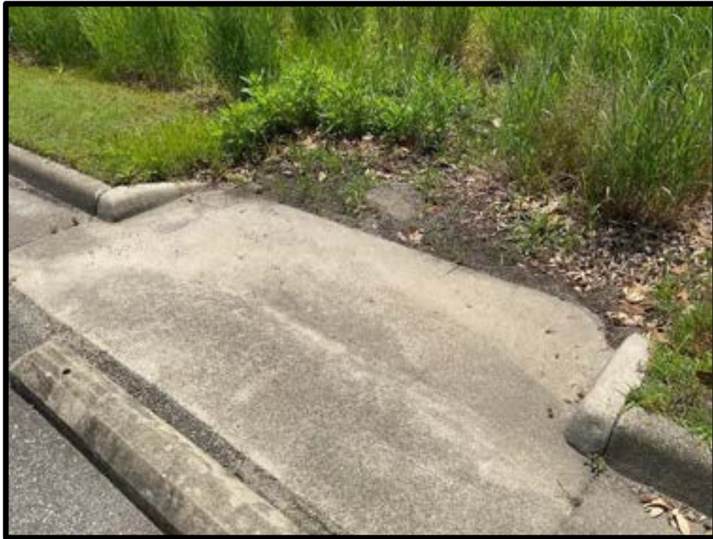
Photo #2: Some sediment accumulation present in northwestern curb cut inlet
